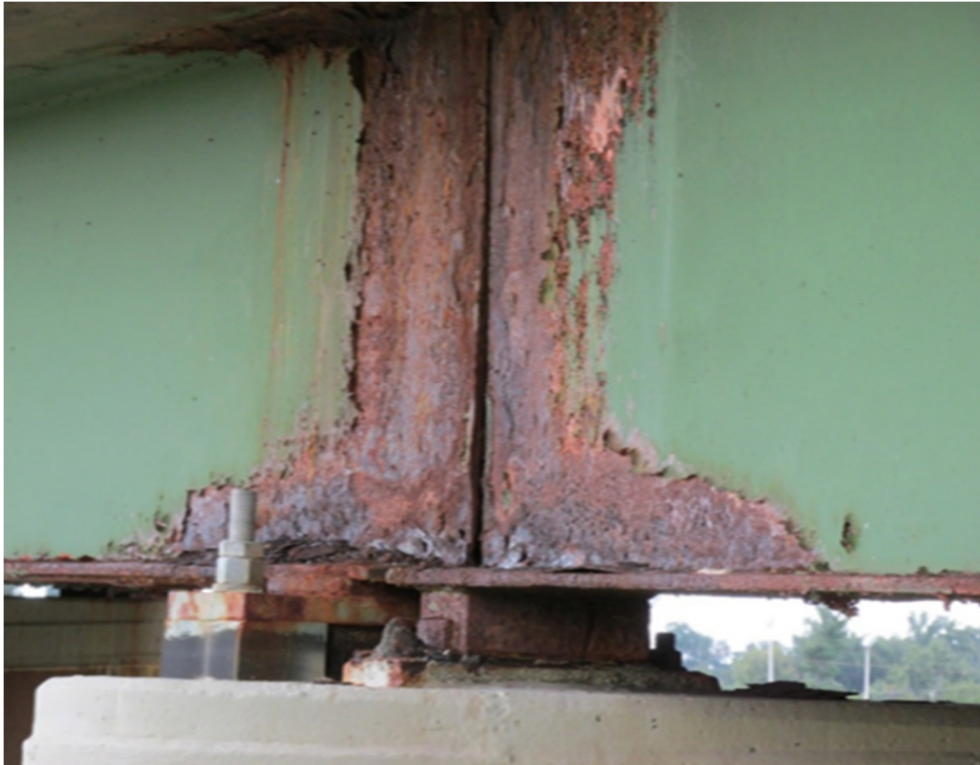
Figure 2: A common observation in the field is that salt-laden water leaking through the expansion joints in bridge decks leads to coating damage and corrosion-related section loss, which is located almost exclusively at the beam-ends
