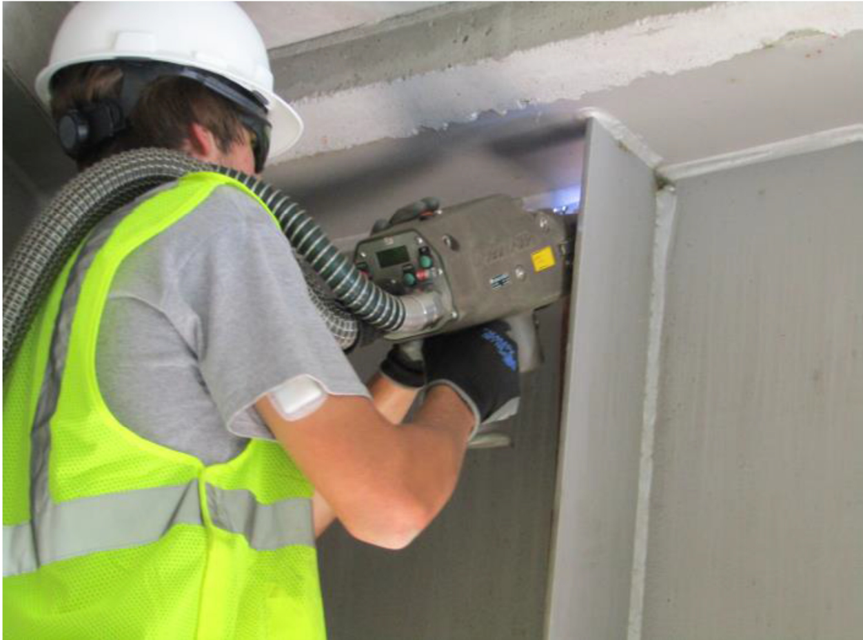
Figure 6: Photograph showing laser ablation coating removal (LACR) on an interior plate girder of an in-service bridge
