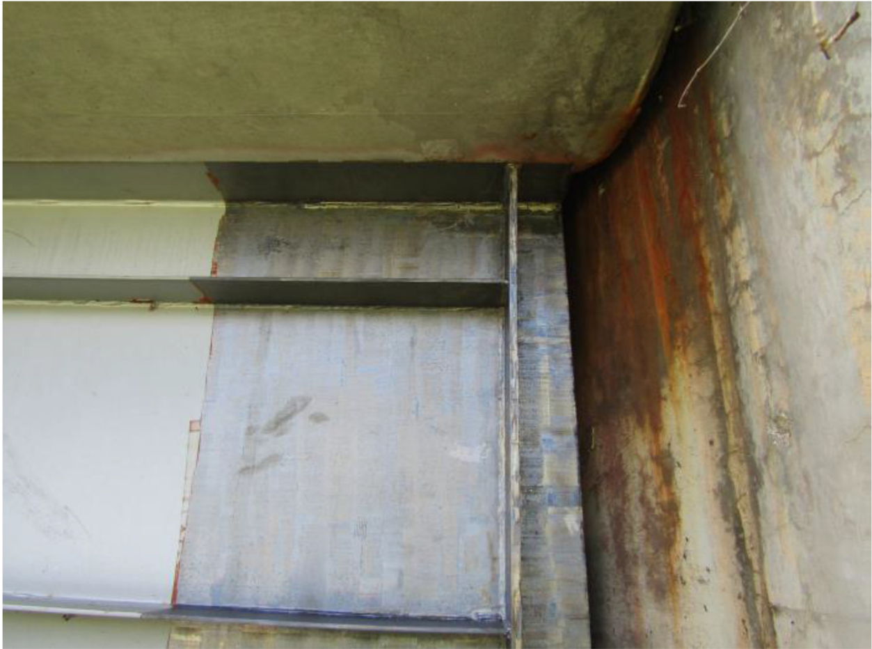
Figure 7. Photograph showing the plate girder after laser ablation coating removal LACR has removed the coating and a clean steel surface is ready to be recoated
